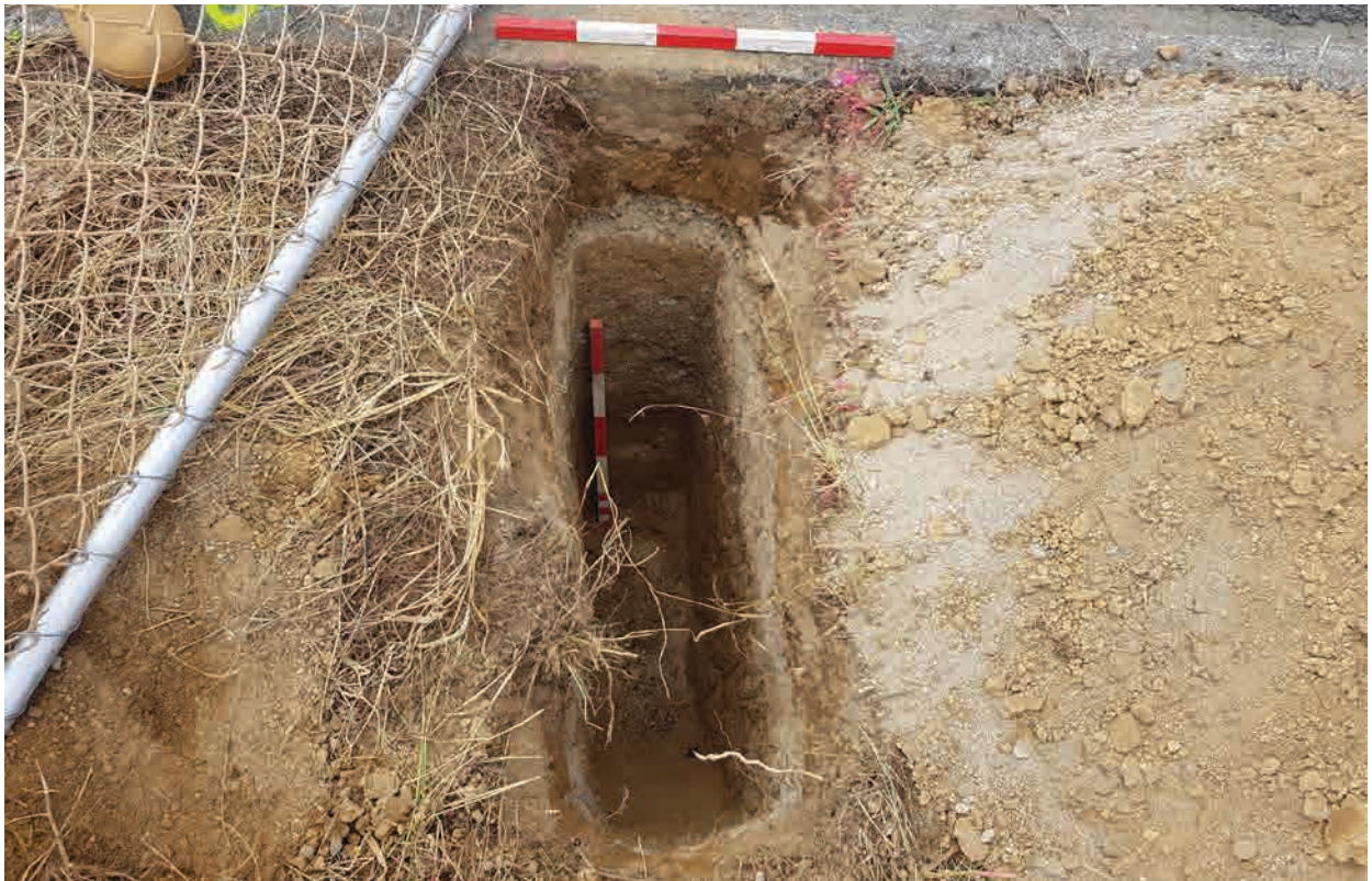
Figure 4. Pothole on Leslie Street showing metal road beneath current street surface. Photo scale = 0.5 m.
