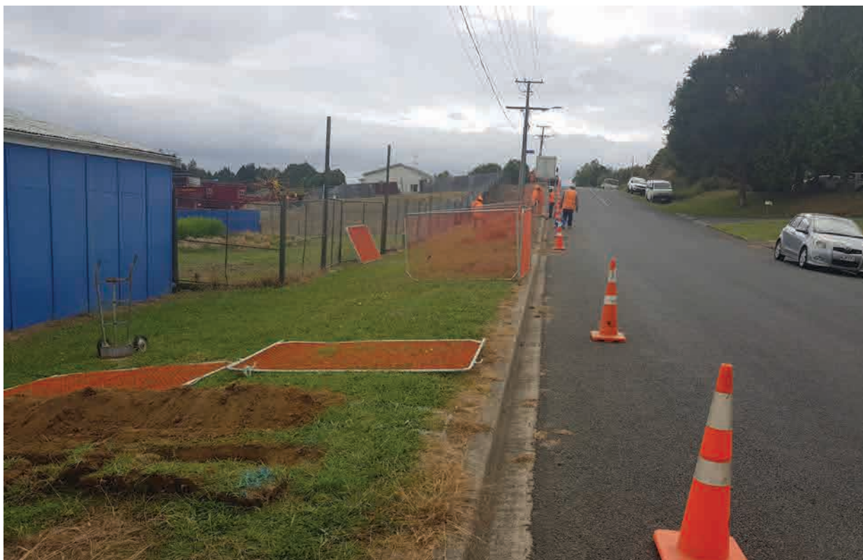
Figure 3. Leslie Street showing lateral potholes to expose existing services prior to a drill shot.
